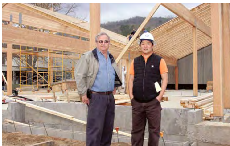
Construction is under way on the Education and Research Wing at the Museum of the Cherokee Indian. Pictured here are Ken Blankenship (left) of the Museum and Steve Ahn, construction project manager
